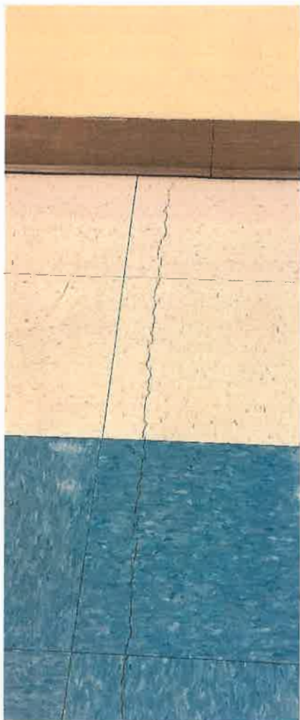
VCT tile cracking (condition typical throughout building)
