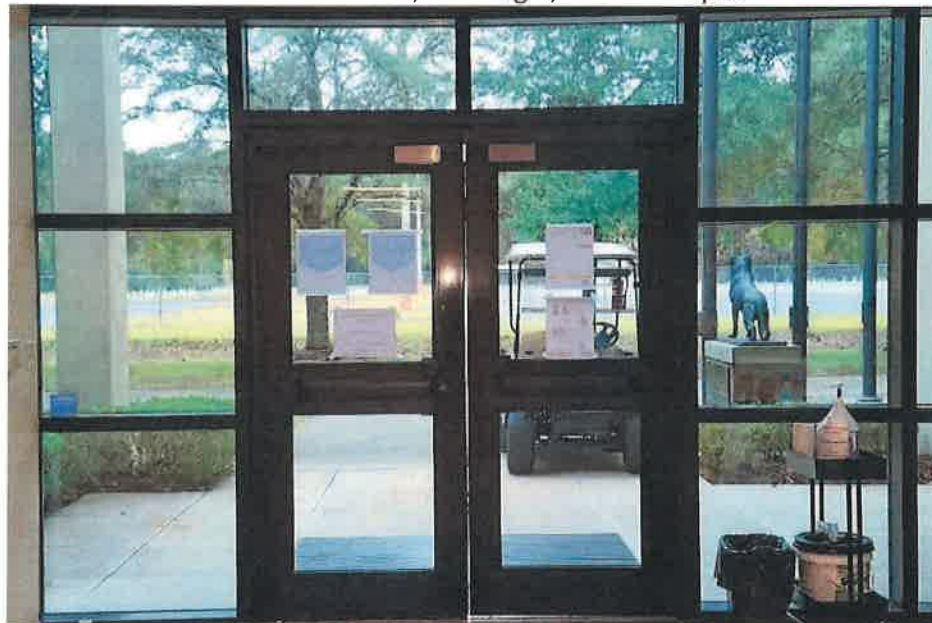
Gaps in doors caused by destabilization of the building slab.
