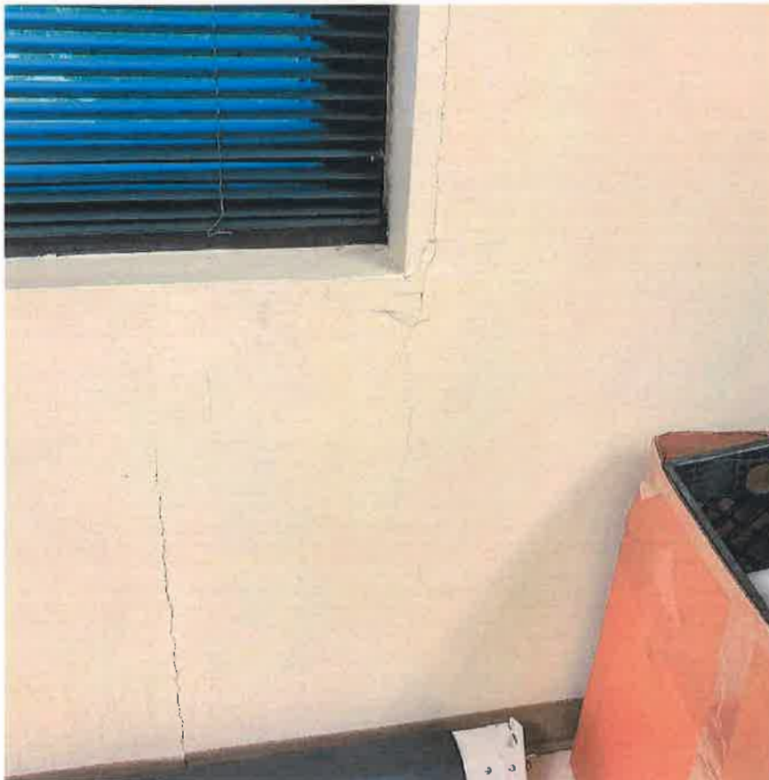
Cracks in sheetrock and frames of windows (typical condition throughout building)
