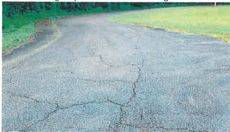
Emergency Vehicle Driver Training Track (condition typical throughout track)
