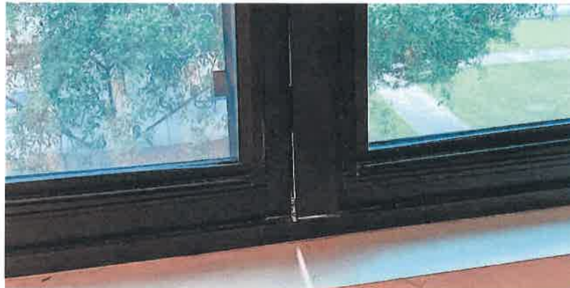
Window frame separation
